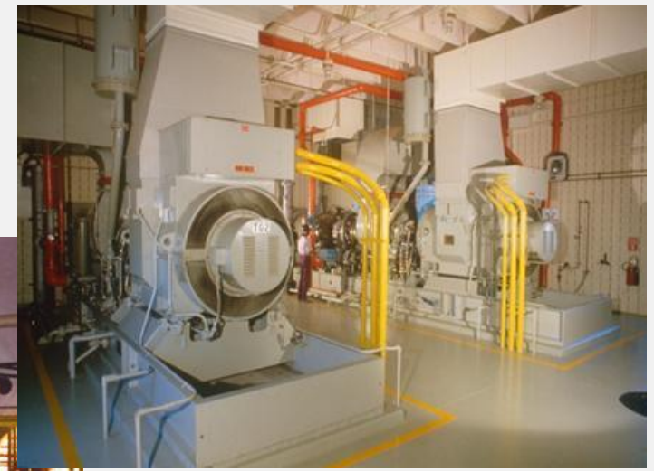
Solar 3 MW Gas Turbine Milwaukee, WI
