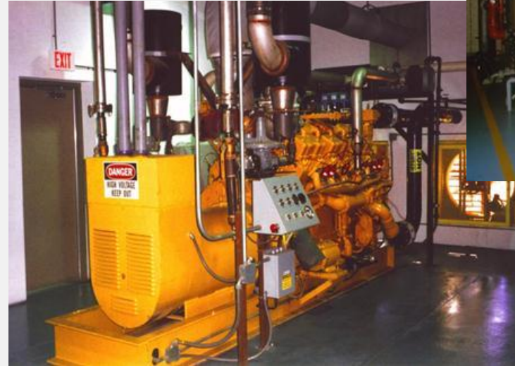
Caterpillar 3516 800 kW Genset Short Mountain LF Eugene, OR
